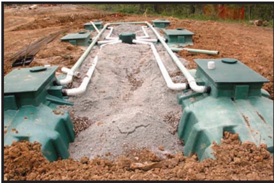
Photo of system for visitor center under construction. Courtesy of Bernheim Woods.
